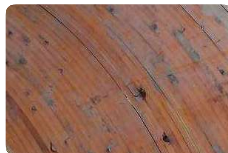
Delaminating cracks © SGI
