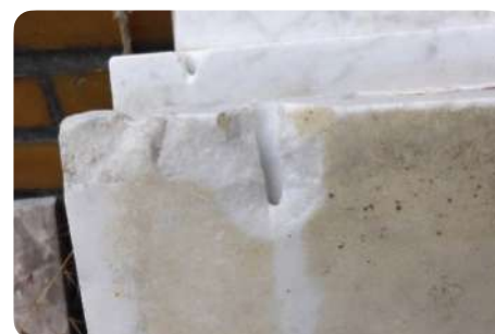
Lug hole enlarged during removal
