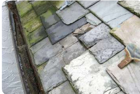
Breaks, cracks and splinters. © nachi.org
