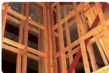
Reclaimed wood frame partitions: 350 m³ of re-claimed timber to create the plasterboard partition structure, BedZED . © Bill Dunster Architects (ZEDfactory, 2002) (UK)
