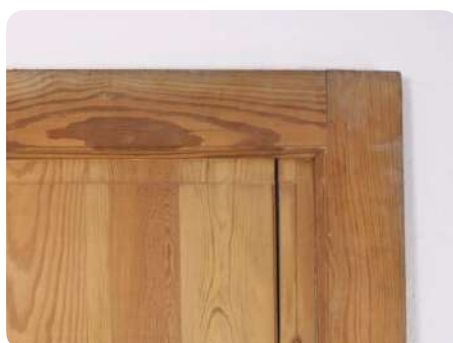
Cracked full panel
