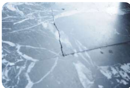
Deep cracks and splinters
