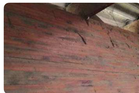
Characterisation of cracks © SGI
