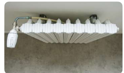
Caserne de Reuilly, Paris Habitat - In situ reuse of 85 cast iron radiators. © ROTOR and SIXIEME CONTINENT
