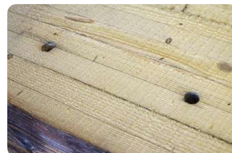
Presence of holes, cracks and damage on the reclaimed elements
