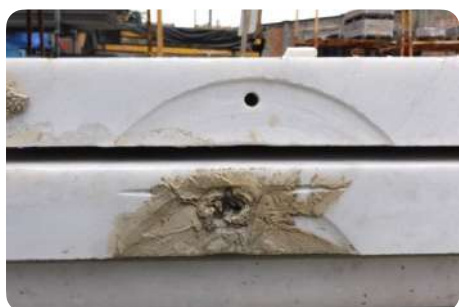
Above: lug hole intact Below: lug hole filled with mortar
