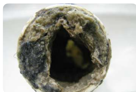
Dirty drainage device
