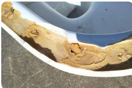
Scaling of the rim and obstruction of the flushing orifice holes
