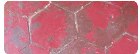
'Prussian Red' paint: warning!
