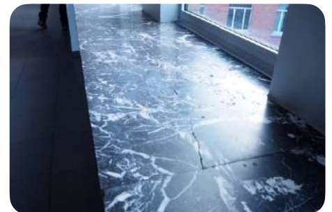
Shelf cracking in its centre
