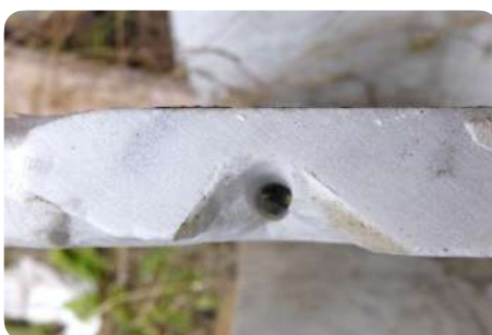
Lug hole enlarged during removal
