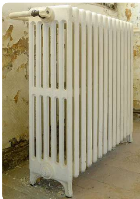
Column radiators - 'Classic' style
