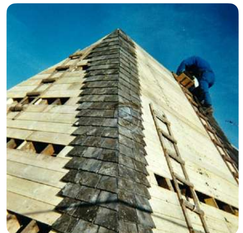
Nailed installation of reclaimed slate, thick model, mixed installation with decreasing gauge (FR) © Sarl Ritouet
