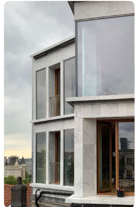
Refitting the slabs on exterior facing, Project Jaspar, Architect Guillaume Sokal, Brussels (BE). © Guillaume Sokal
