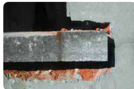
Detachment of the top, side and bottom of the sills © CDR Construction
