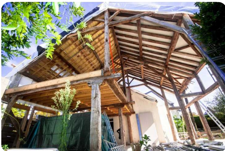
Design of a 110 m 2 residential extension from reclaimed materials, © AASF Atelier Architecture Sarah Fruit, Bati Recup (FR)
