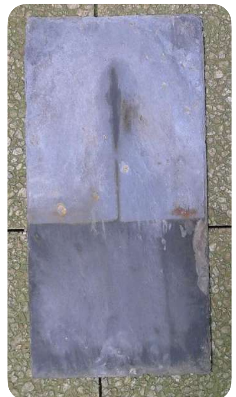
Colour and shade variation between the protected part and the unprotected part © roofslates.com
