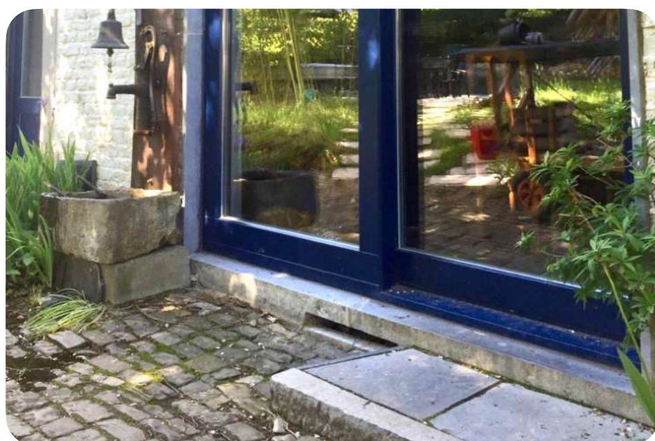
Reuse Inspiration. Sliding sash sill consisting of two old window sills cut to the right size and cut to provide ventilation of the cellar (hole in the centre) © Sophie Boone
