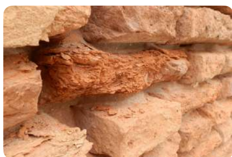
Crumbling brick, unsuitable for reclamation
