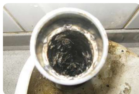
Partially cleaned drainage device
