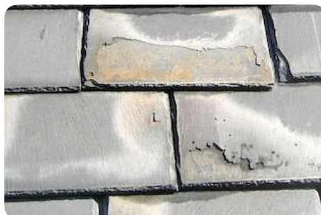
Efflorescence and delamination. © nachi.org
