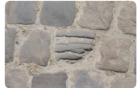
Example of a poorly laid sandstone sett. The cleavage plane must be parallel to the direction of laying. In this case, the sett probably underwent stresses which caused its cleavage. This sett will be discarded during sorting related to reclamation.
