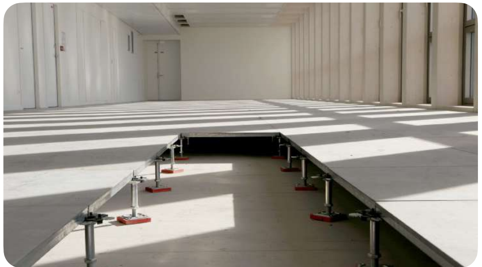
Re-installation of raised floor coverings and new jacks (FR). © Mobius - Marie Moroté
