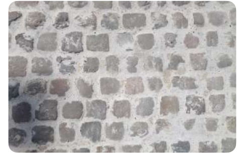
Setts with cement joints: recovery promises to be difficult
