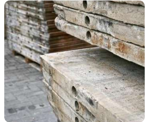
Panels before treatment
