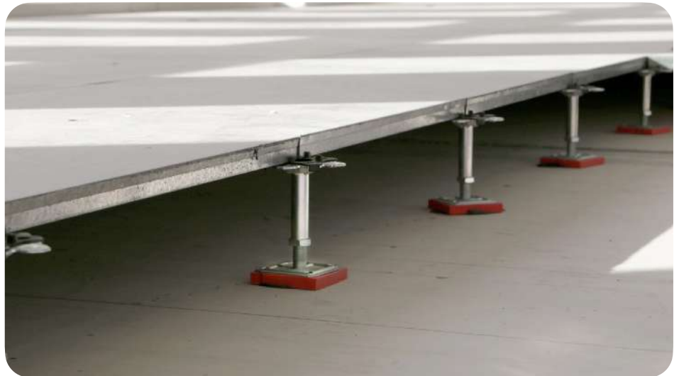
Re-installation of raised floor coverings and new jacks (FR). © Mobius - Marie Moroté
