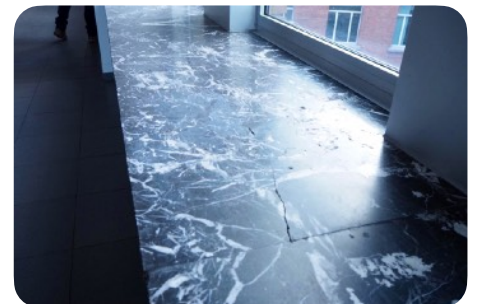
Shelf cracking in its centre
