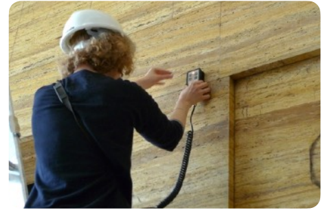
Searching for metallic anchoring elements of a natural stone facing using a pachometer. © CSTC
