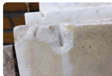
Lug hole enlarged during removal
