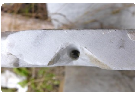
Lug hole enlarged during removal
