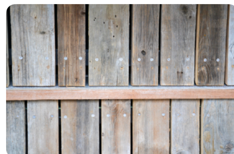
Installation of 2600 m 2 of barnwood cladding from Eastern Europe, Institute of Botany of the ULg, Liège (BE) © André Warnier
