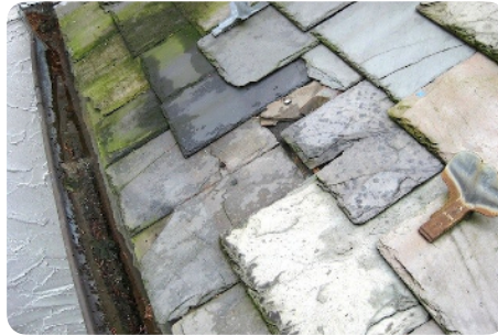
Breaks, cracks and splinters. © nachi.org
