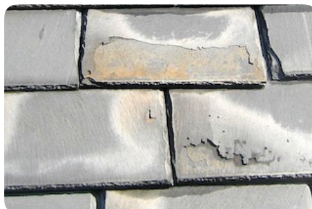
Efflorescence and delamination. © nachi.org
