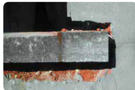
Detachment of the top, side and bottom of the sills © CDR Construction
