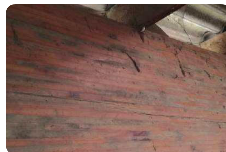
Characterisation of cracks © SGI
