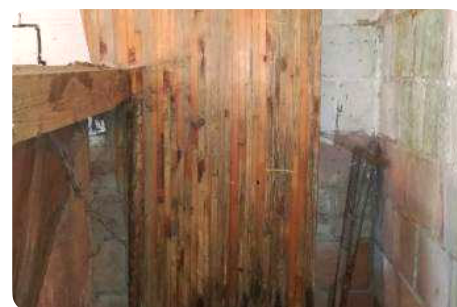
Deterioration due to prolonged exposure to humidity © SGI
