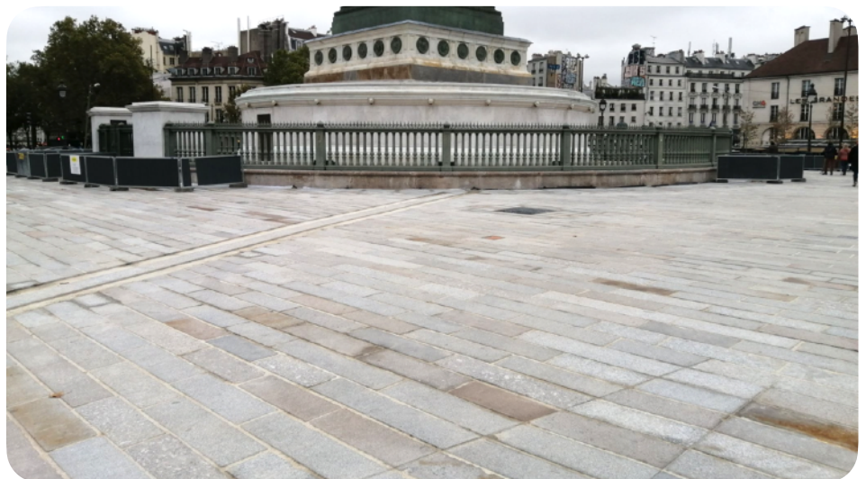
Place de la Bastille, Paris. Reclamation of 10,000 old kerb stones sawn in half to be transformed into flagstones (FR). © Benjamin Randow
